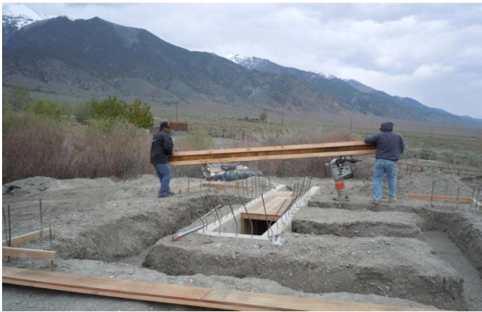
Photo #1 Cutline: Workers help construct the Kingston Creek Hydro Project, which is fed from a year round stream source in the Big Smoky Valley.
