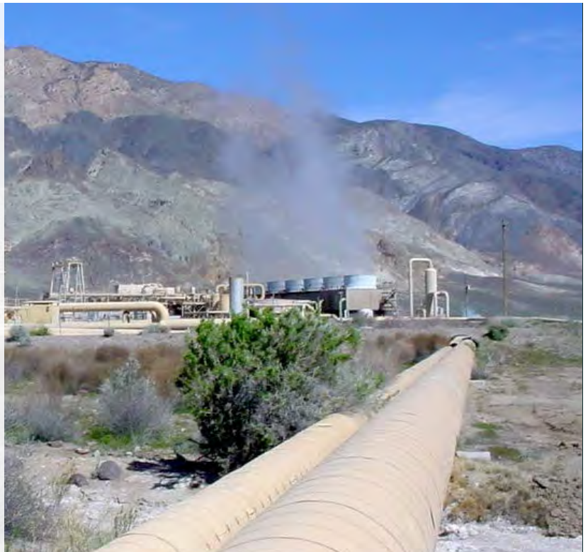
At 67 MW, the Dixie Valley geothermal facility is the largest individual geothermal plant in Nevada. Photo courtesy of Terra-Gen power.
