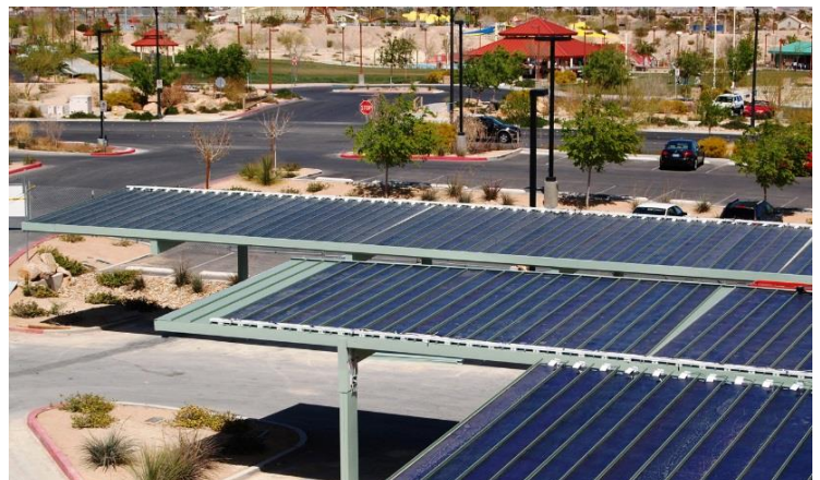
Figure 1. A GOE loan funded three City of Las Vegas solar parking shade structures. City of Las Vegas received $1.2 million from the Governor's Office of Energy to build the structures, which created 12 construction jobs, produced 1.2 million kWh of electricity annually, and reduced carbon emissions 23.8 million pounds of CO 2 during the first 20 years of operation.
