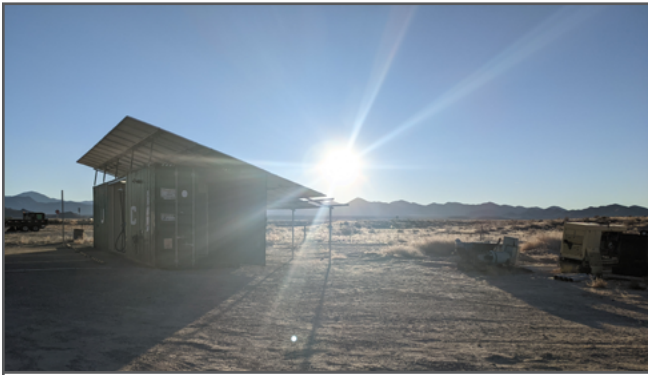
Solar panels and an electric vehicle charging station at Middlegate Station, on U.S. Highway 50 about 50 miles east of Fallon. Photo courtesy of Howard Construction.
