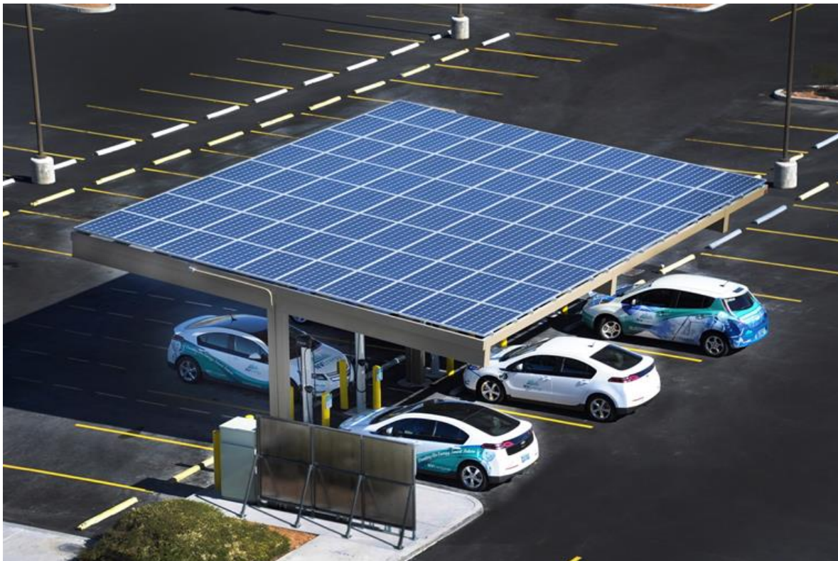
Solar PV powered charging stations at NV Energy's Pearson Office Building in Las Vegas. (Photo courtesy of NV Energy.)
