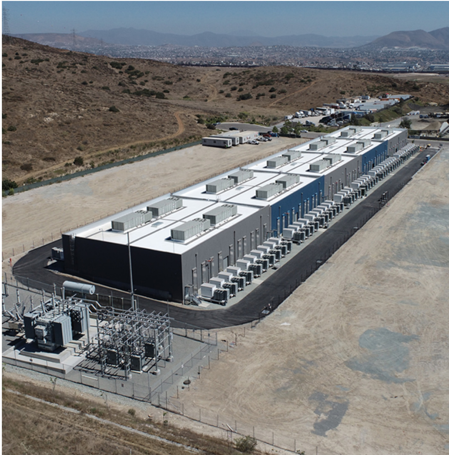
Gateway Energy Storage in Otay Mesa, CA 250 MW, operating since August 2020
