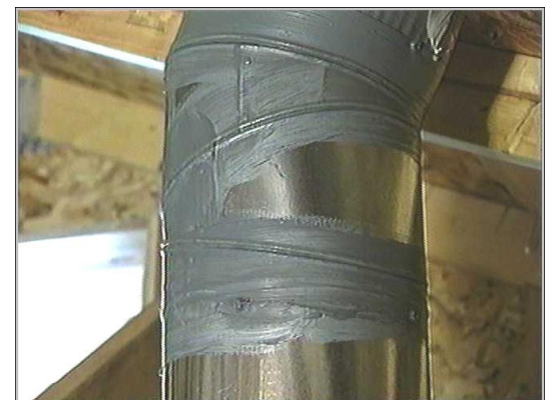
This duct has been sealed but not insulated
