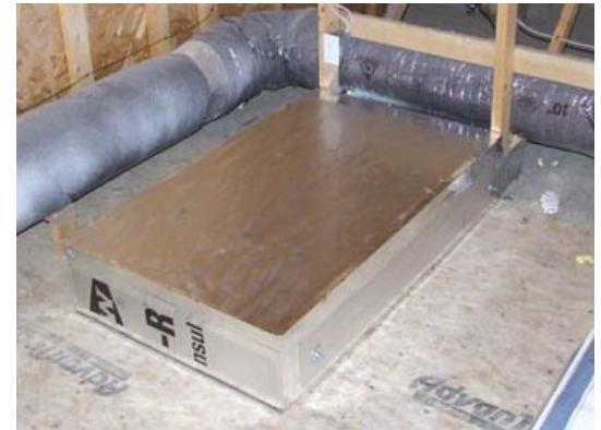
Insulated attic hatch and insulated ducts
